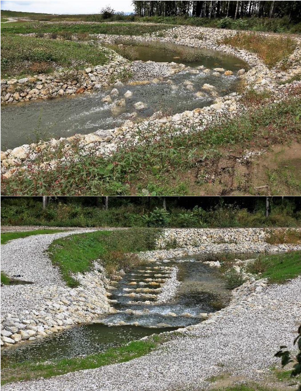
Figure 34: HPP Brežice and the fish pass on the Sava River one year after construction
